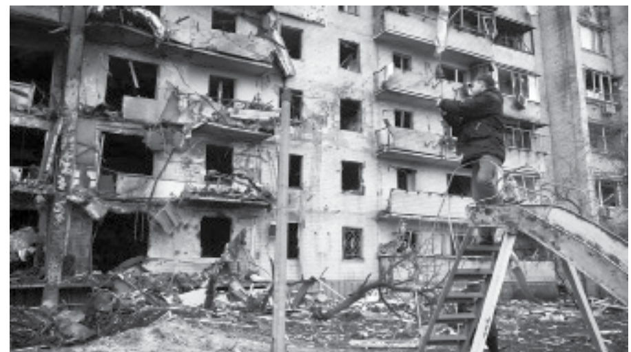
© UNICEF/Anton Skyba for The Globe and Mail | A man photographs an apartment building that was heavily damaged during escalating conflict, in Kyiv, Ukraine. Photo from UNCTAD website.
